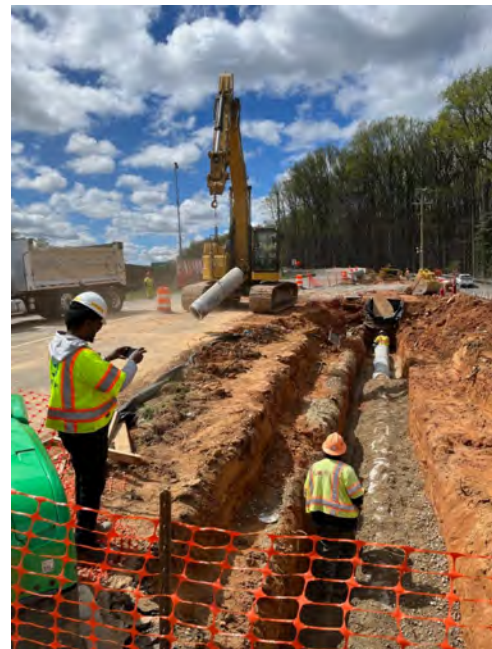
Adjacent to the Langley Swim and Tennis Club, an excavator lifts a segment of drainage pipe (April 5).
